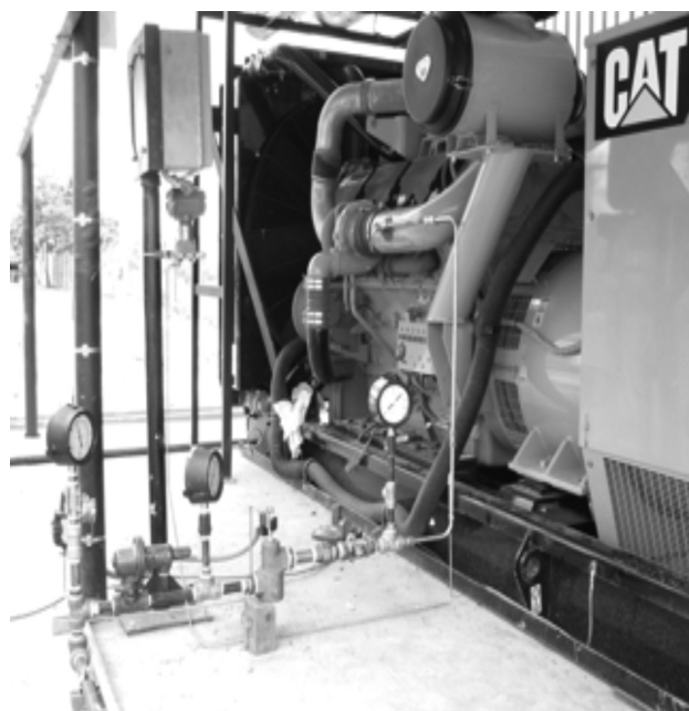
Figure 4. Power generator set used.
